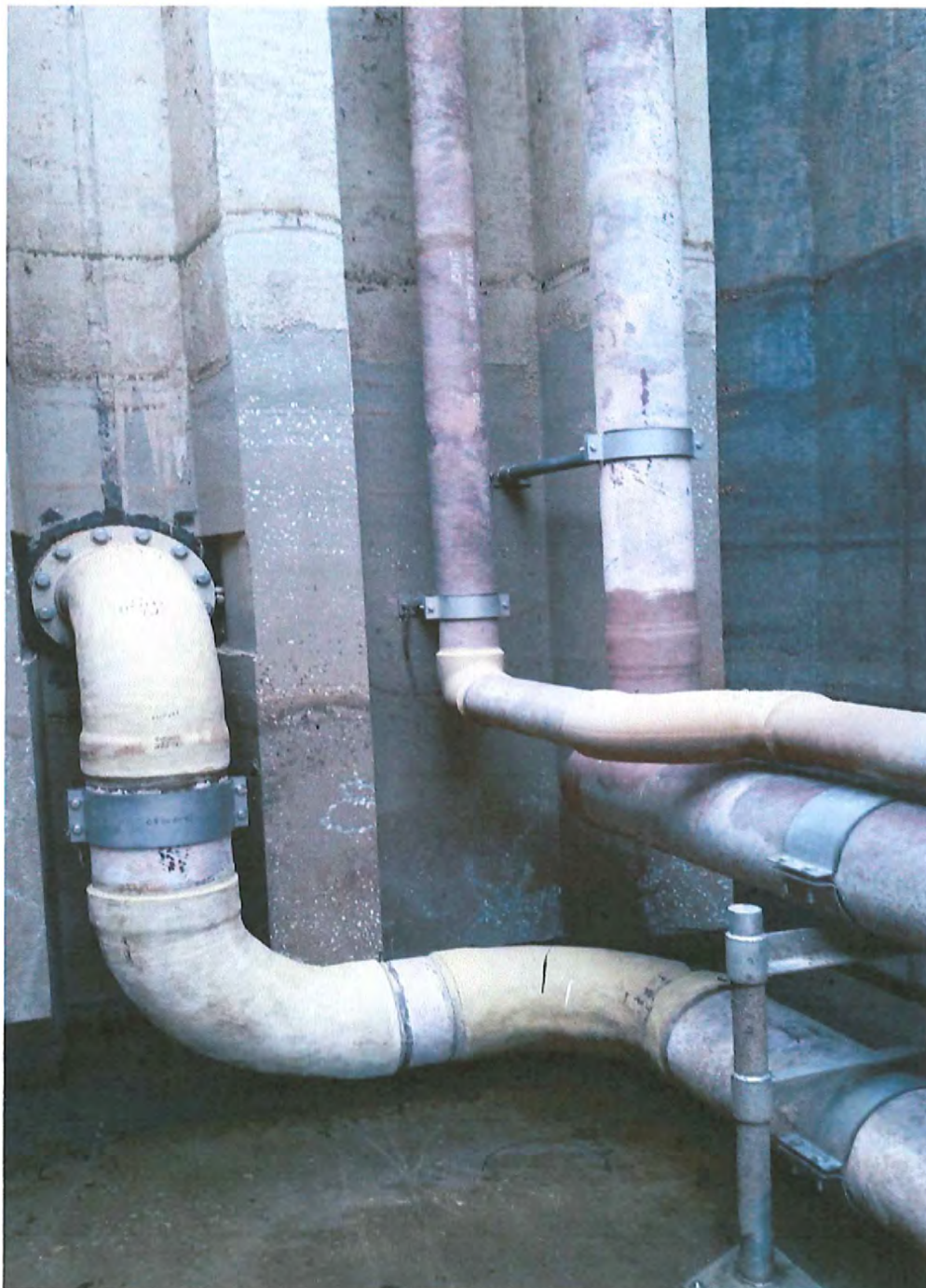
Figure 2 - Influent and Aeration Piping
