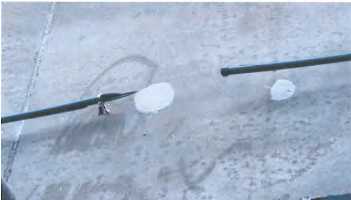
Figure 5 - Broken Aluminum Sulfate Solution Conveyance Pipe
