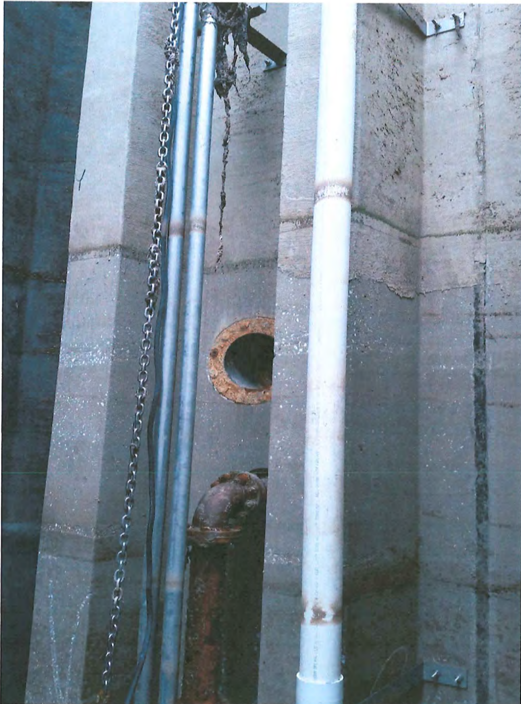
Figure 4 - View of Sludge Waste Pump Guide Rails, Discharge pipe and Visible Concrete Aggregate
