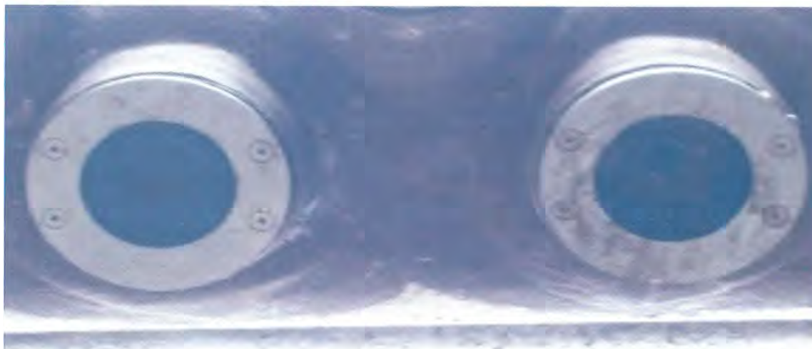
Figure 1 - SBR 2 Failed Decanter Valve (right side)
