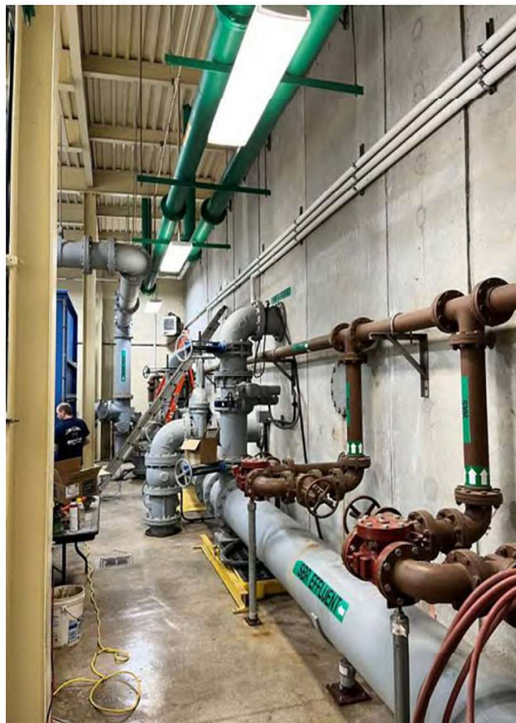
Pipes, pumps and system maintenance
