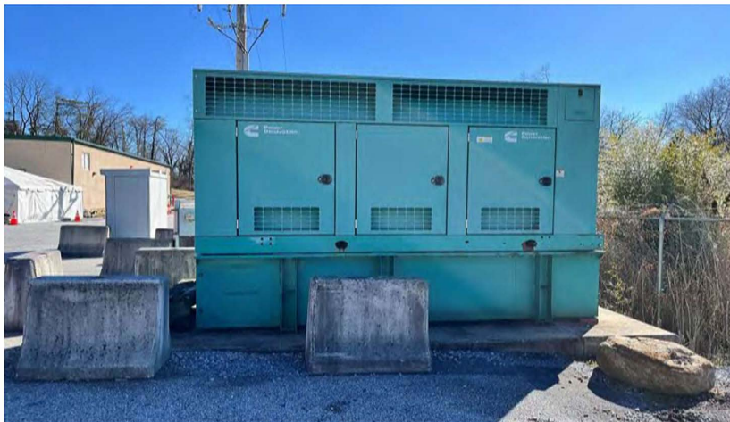
Backup power supports reliable sewer operations
