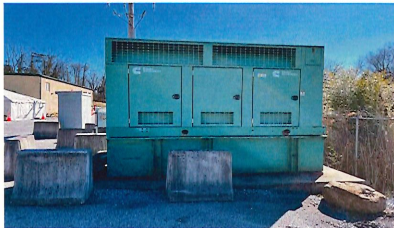
Backup power supports reliable sewer operations
