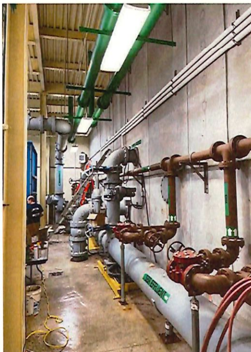
Pipes, pumps and system maintenance
